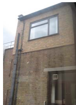
The rear façade of 186KPR showing the different bricks used for the external wall of the 2001 roof extension. Note the modern window openings in the masonry walls of the extension and 2 nd floor
