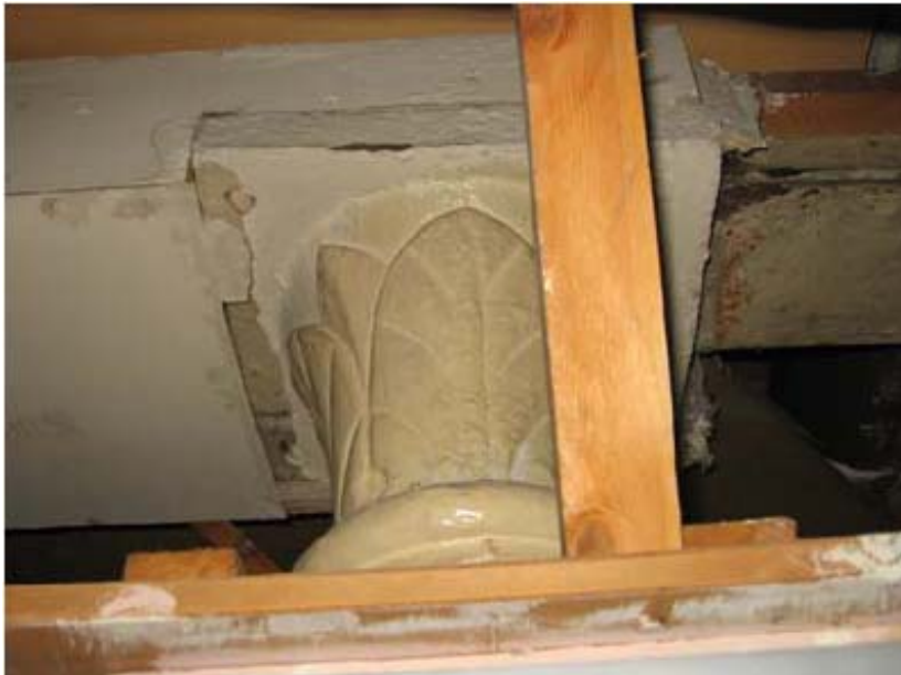
Photograph showing the head of column on ground floor of 18aSS supporting the first floor steel beam structure above
